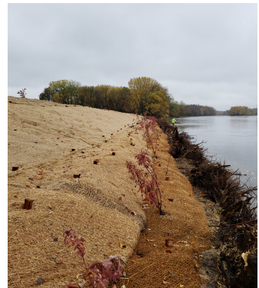
Native plants, seeding, erosion control blanket, and toe-wood installed on finished project.
