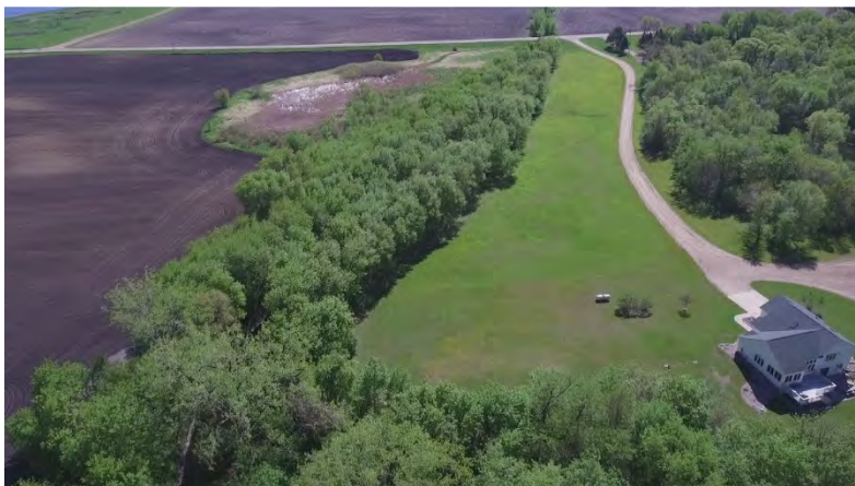
Figure 24. Clearing and Grubbing Tree Removal Southeast Quarter of Section 12 of Stockholm Township
