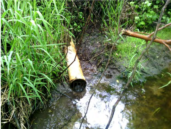
Figure 40. Unprotected Tile Draining into the Main Open Ditch
