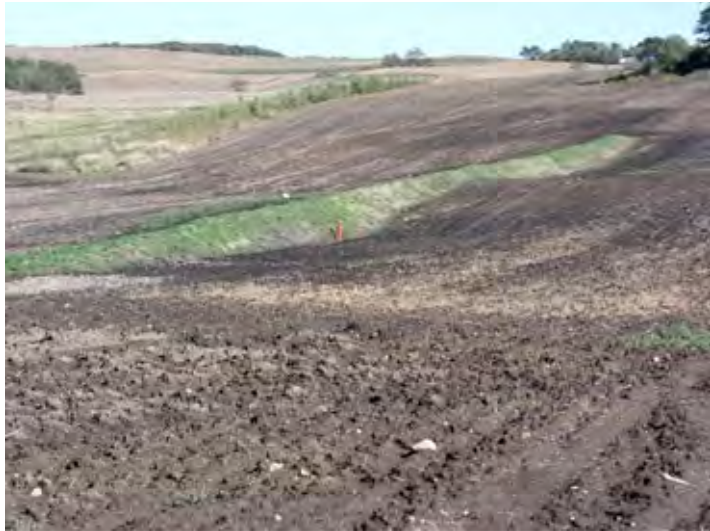
Figure 46. Typical Constructed WASCOB
