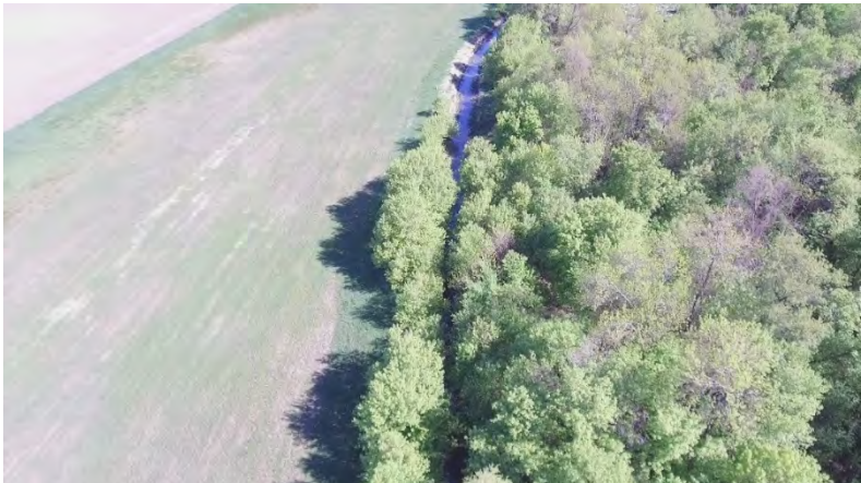
Figure 28. Clearing and Grubbing Tree Removal Northeast Quarter of the Southwest Quarter of Section 24 in Stockholm Township on Sieg Lateral
