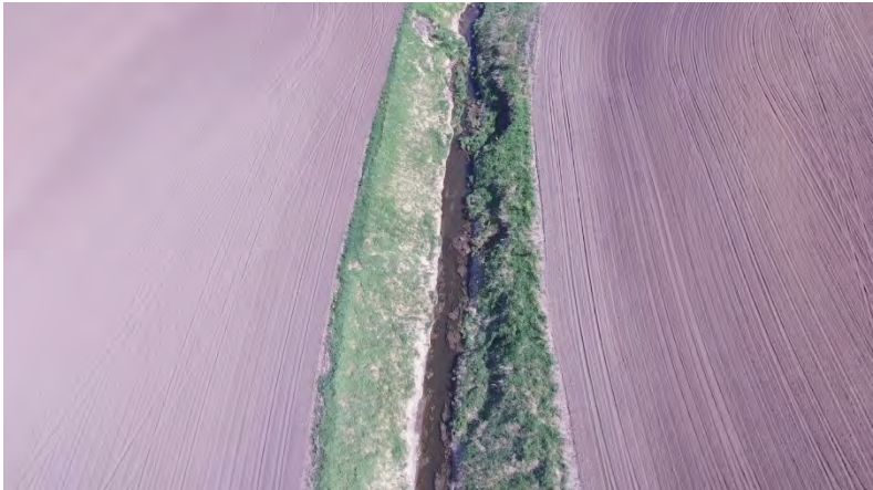
Figure 32. Sloughing along open ditch in the Northeast Quarter of Section 24 in Stockholm Township on Sieg Lateral
